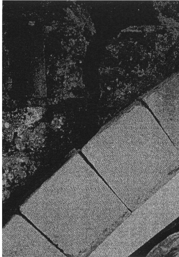
Fig. 2.7 Clare College 1 Bridge, Cambridge. Another view of the region shown in Fig. 1.5. The increase in span of the central arch has led to the formation of hinges between voussoirs.
