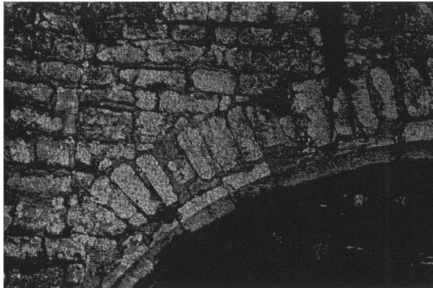
Fig. 5.4 Rough masonry of Teston Bridge, Kent, forming an arch ring of about 200-400 mm.
